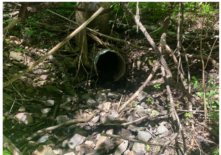
Figure 1. EJCT 055 is eroded, perched and undersized.
