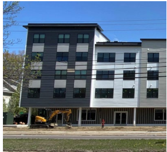
Figure A, above left: Western portion of the building as permitted in 2017. Figure B, above right: Western portion of the building as built.
