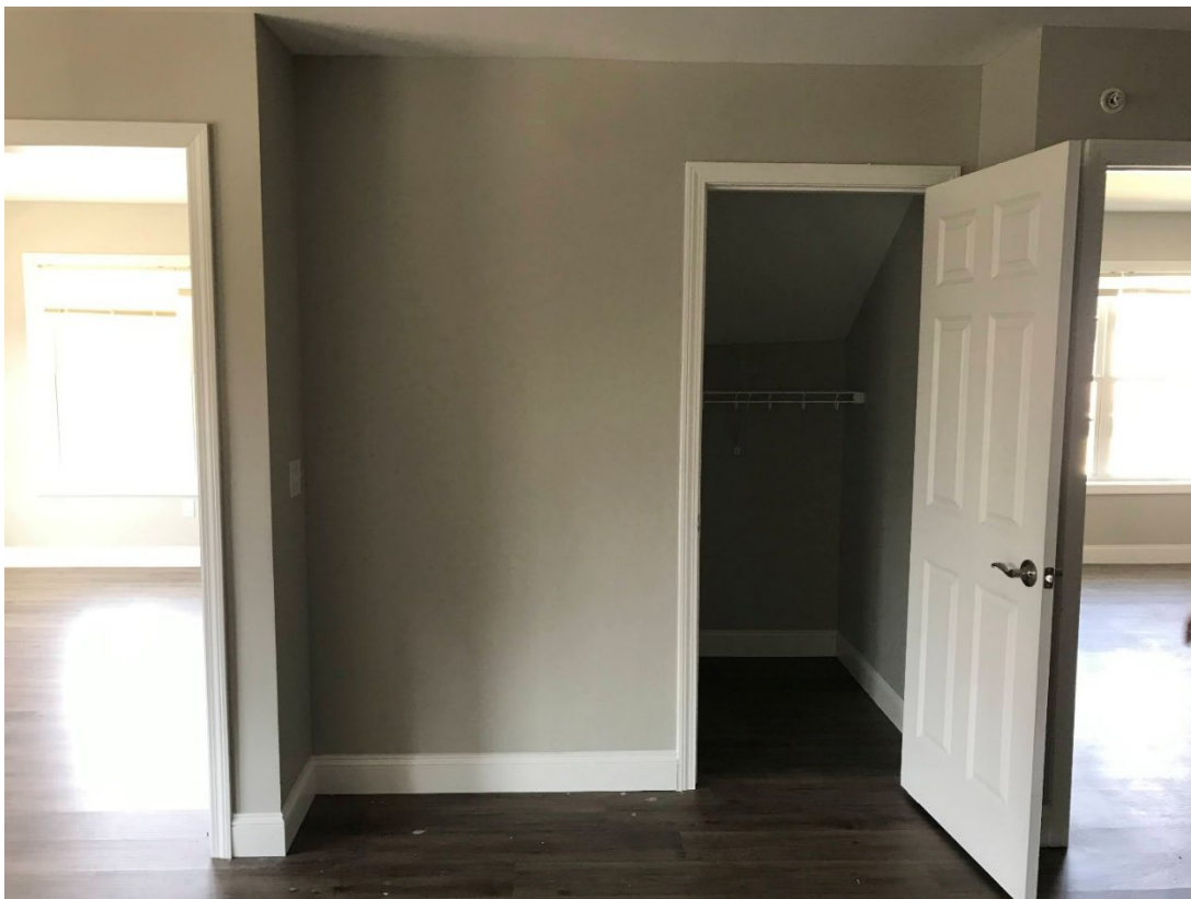
Figure C: Unit 413 during the Certificate of Occupancy walkthrough. The stairs leading to the fifth floor are sealed off by the constructed wall located directly to the left of the doorframe.
